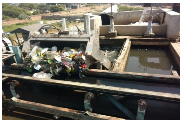
Figure-5: Screening Chamber at STP, Sajidhera.
