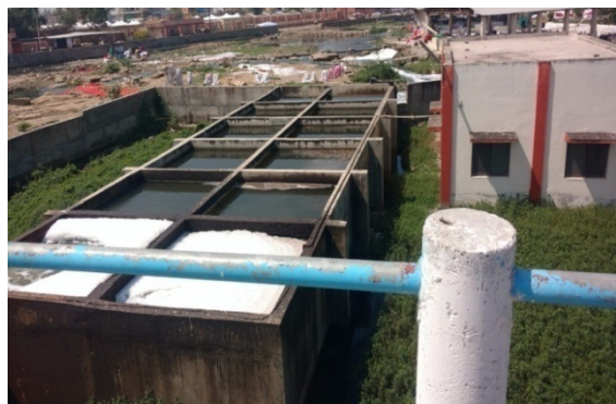
Figure-7: Outlet Chamber at STP, Sajidhera.
