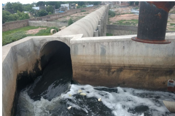
Figure-4: Inlet Chamber at STP, Sajidhera.
