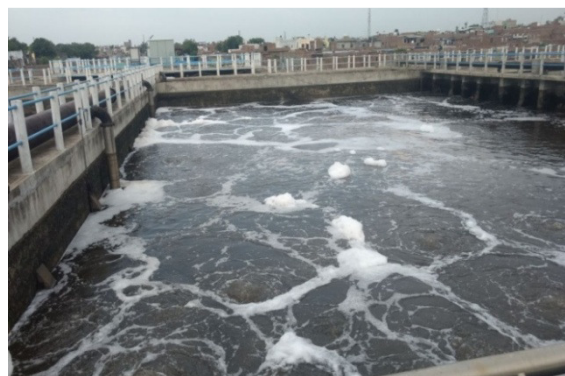
Figure-6: Sequential Batch Reactor (SBR) at STP, Sajidhera.
