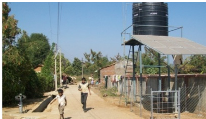
Figure-3 Solar energy based dual pump drinking water supply scheme in Nagpur, central India
